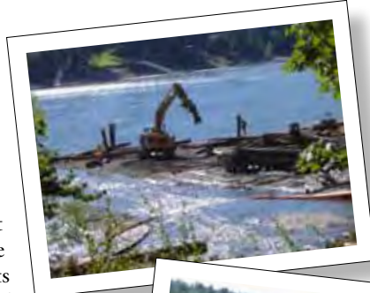
Secured logs are stacked around wood pilings in the gravel at the mouth of the creek.
