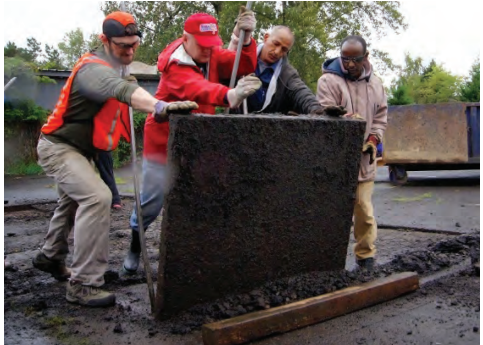
Volunteers came out in force to remove asphalt, condition the soil, and install 500 native plants at St. Mary Ethiopian Orthodox Church this fall.
