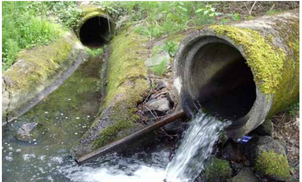
Artificial obstructions such as culverts, bridges, dikes, dams and road fills are common examples of structures that limit or exclude fish migration into more preferable habitats. Butler Creek culverts, above.
